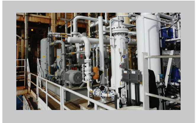
Xebec's compact M-3100, fast cycle PSA was the perfect footprint for the off-shore Platform Gail in Santa Barbara
