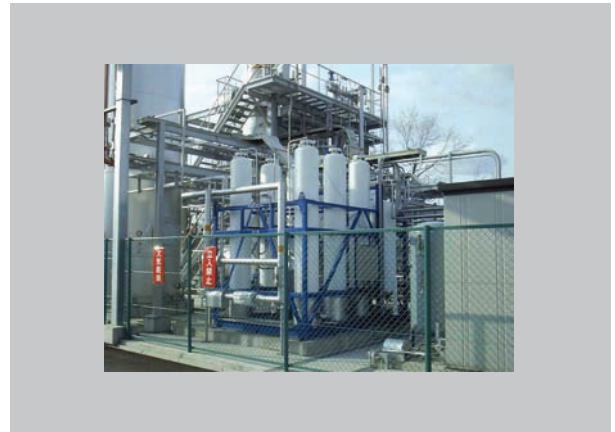
XEBEC's compact, fast-cycle PSA systems and their reliable rotary valves proved a perfect fit for MKK, Ltd. in Japan.
