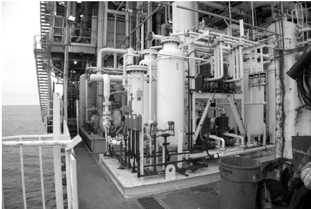
Figure 6. Photograph of Entire Xebec Rotary-Valve, Fast-Cycle Pressure-Swing Adsorption Unit On-Board Platform Gail (note – above rotary valves)
