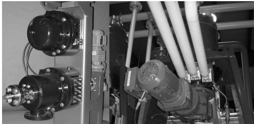
Figure 2. Detailed Photographs of Heavies/Lights Xebec Rotary Valves
