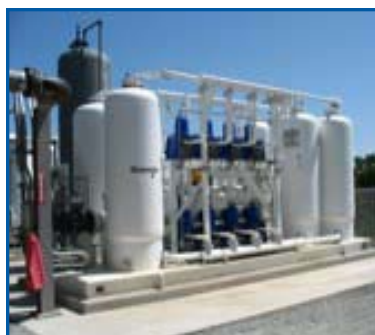
Biogas purifiers for biogas upgrading
