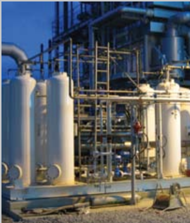
XEBEC H-3100 2700 Nm 3 /hr unit at HydroEdge liquid hydrogen plant in Japan.
