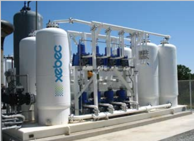
XEBEC M-3100 processing landfill gas in Ohio for distribution to customers via Duke Energy natural gas pipelines.
